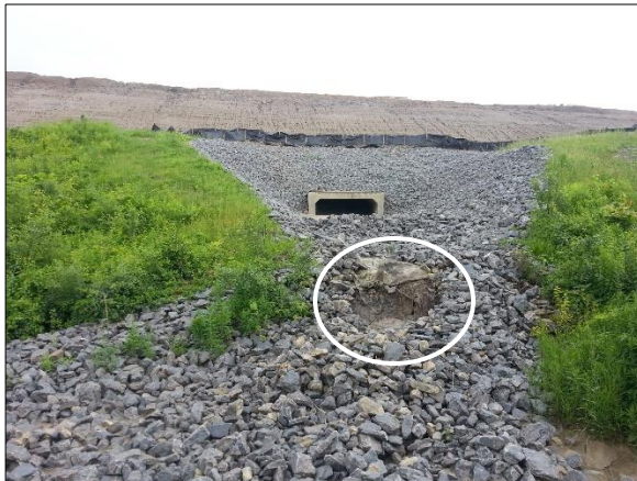
Photo 4a. Storm flow out of a 1.5m high box culvert conveyed the riprap armour and ripped the geotextile.
