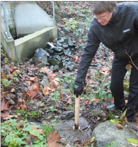
Photo 2. Water flow below geotextile
