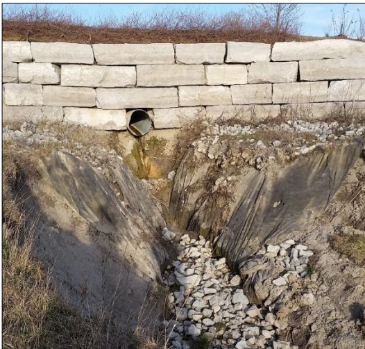
Photo 1a. Apparent storm flow failure
