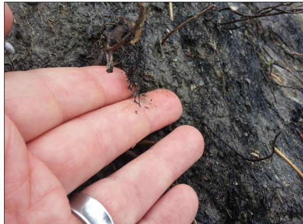
Photo 4b. Grade remained stable because of remnant shrub rootzone left in place below the geotextile.
