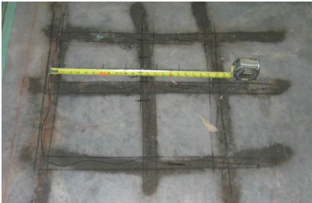
Figure 2: Sample markings identifying embedments in concrete with appropriate exclusion zone
