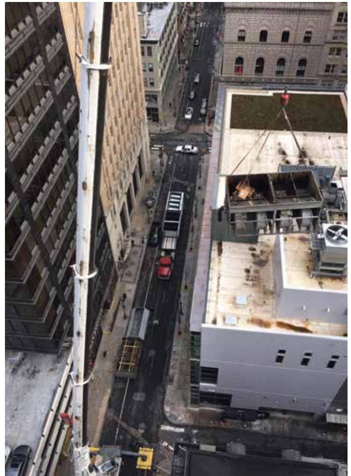
Photo credit: West Chester Mechanical
