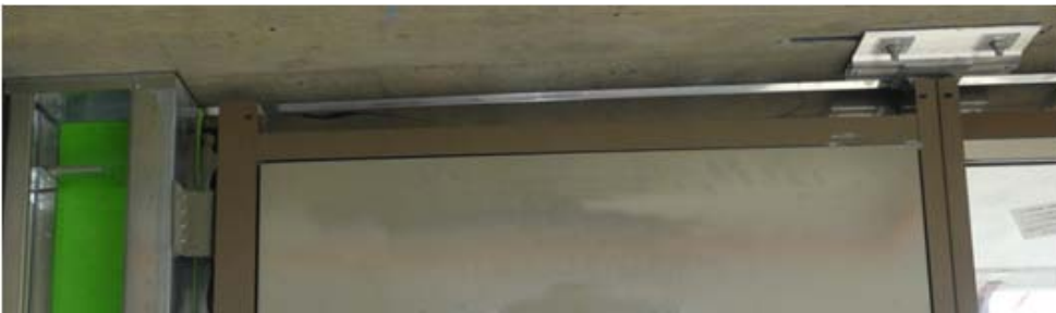
Figure 11. Interior photograph of the head of exterior wall. Indirect support of a glazed curtain wall jamb mullion through an adjacent light gage metal framing. (Note the stub of the single deflection track on the left side.)
