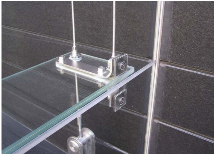
Figure 1. Example of the vocabulary challenge. The structural glass wall, with horizontal structural glass mullions suspended on stainless steel cables. The glass fins play structural role by resisting lateral load, as opposed to the traditional load-collecting role of glass. No structural sealant used here.
