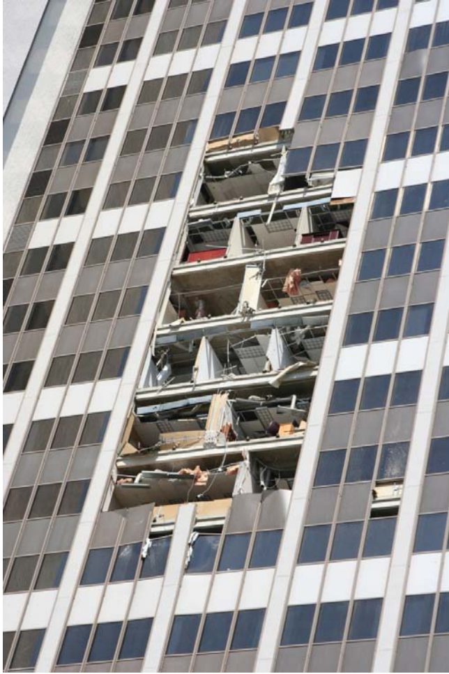
Figure 12. Exterior photograph of exterior wall. A spectacular, catastrophic collapse resulting from uncoordinated support of a curtain wall.. Jamb aluminum mullions were exclusively supported onto adjacent CMU piers, which had insufficient load resistance to collect design reactions from the curtain wall. Photo credit – Mr. Alessandro Abate.
